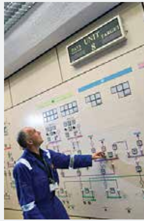
Control room, Heysham Unit 2
